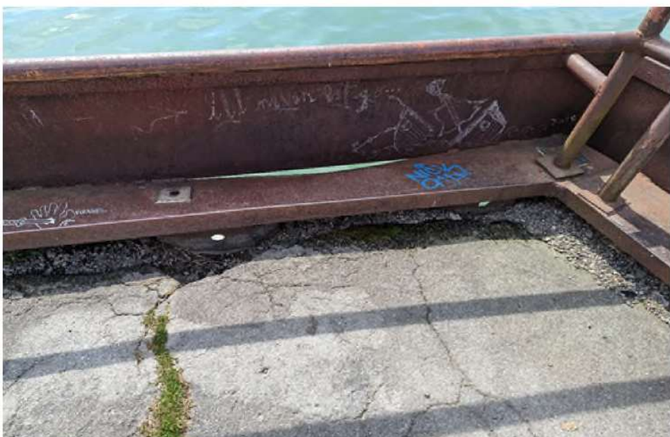
PHOTO 11: DETERIORATED ASPHALT, GRADE SLOPES TOWARD WALL, DAMAGED CAP
