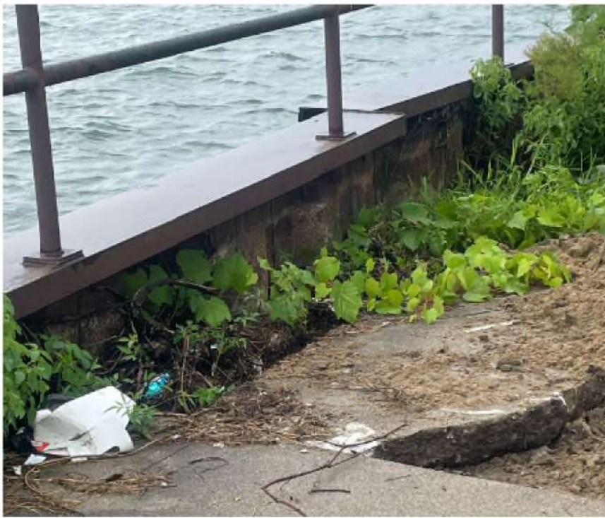
PHOTO 3: SIDEWALK SUBSIDENCE AND OUTWARD ROTATION OF SEAWALL
