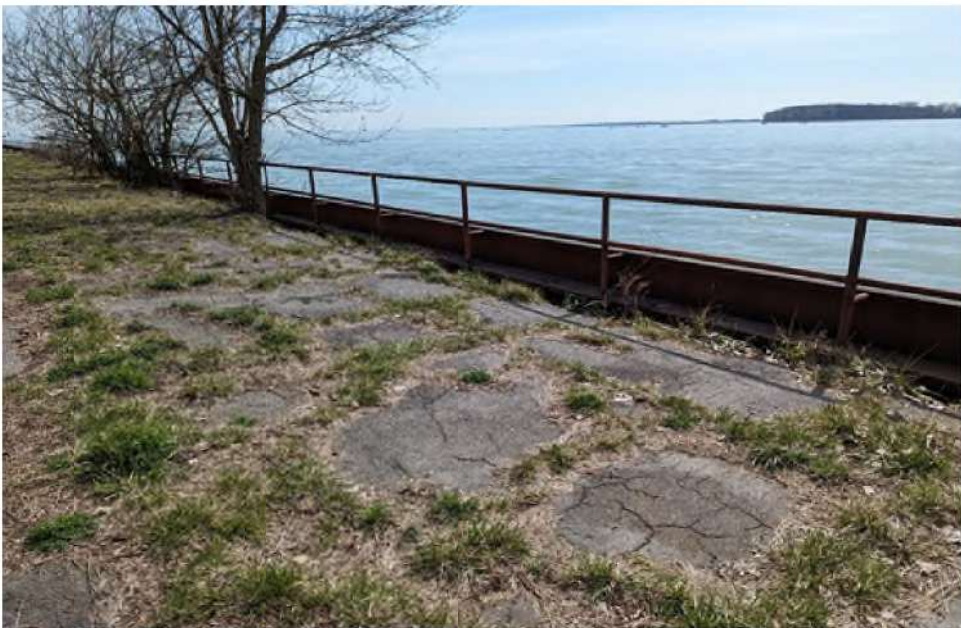
PHOTO 1: DETERIORATED ASPHALT, GRADE SLOPES TOWARD WALL
