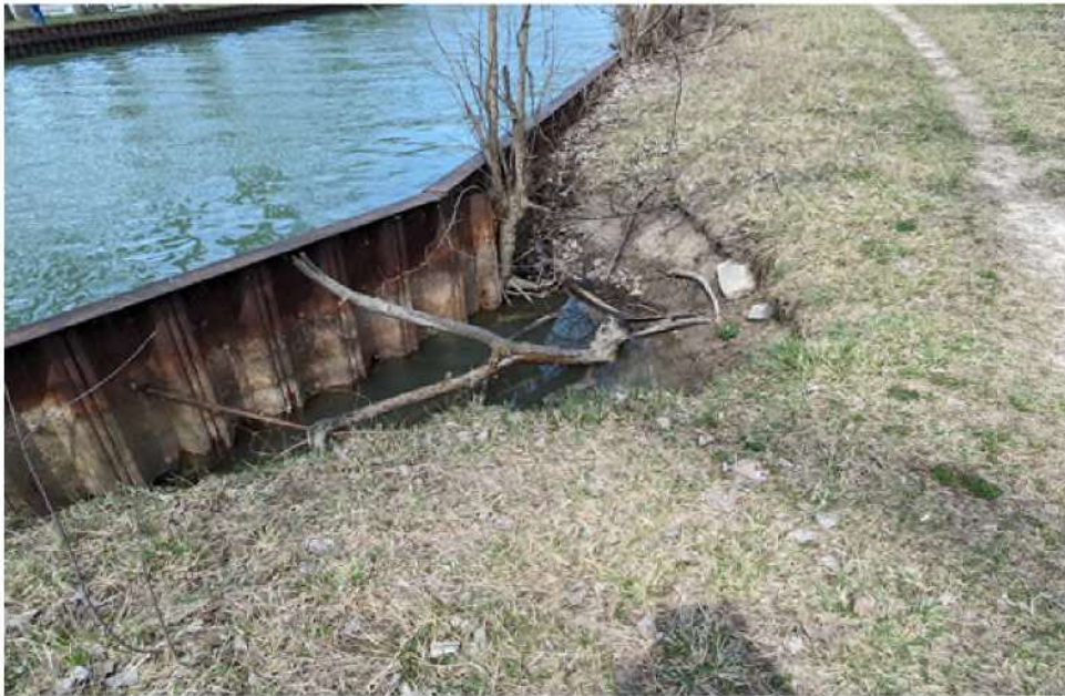
PHOTO 6: BROKEN TIES & EROSION BEHIND WALLS
