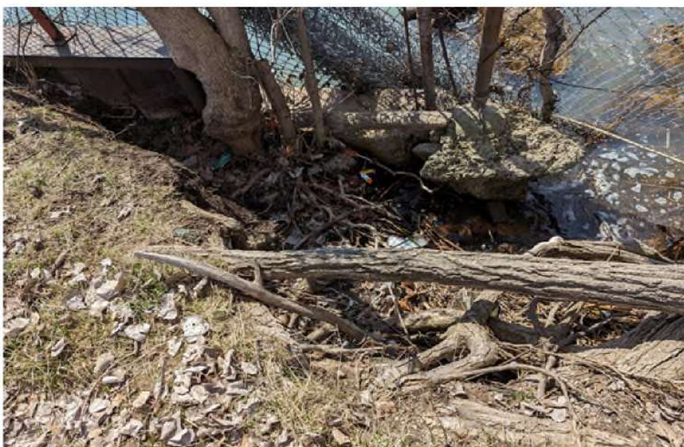
PHOTO 12: TREES & EROSION BEHIND WALL
