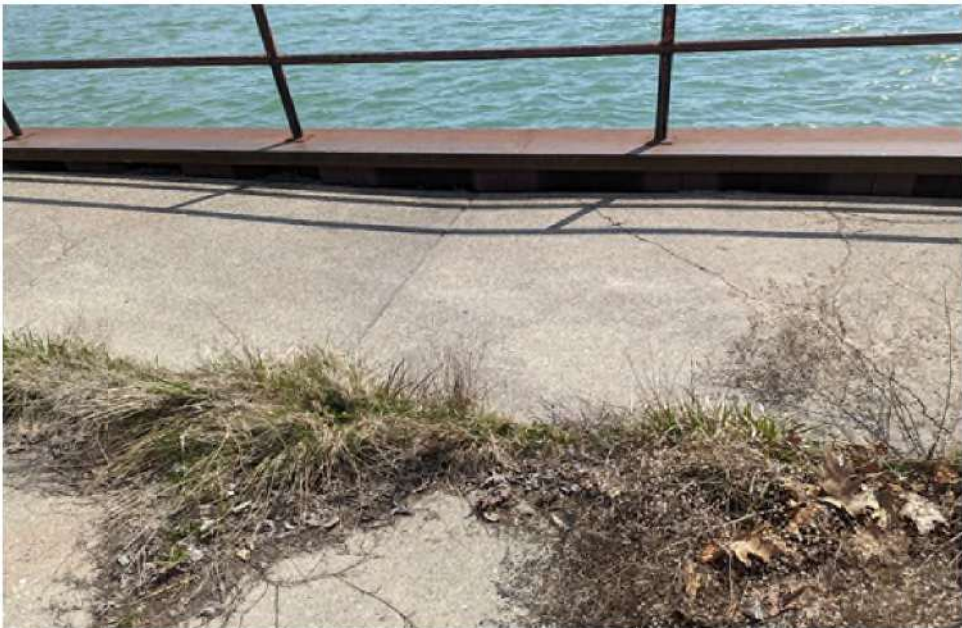
PHOTO 13: "SAGS" IN SIDEWALKS, SIDEWALKS SLOPE TOWARD WALLS, SIDEWALKS NOT MAINTAINED
