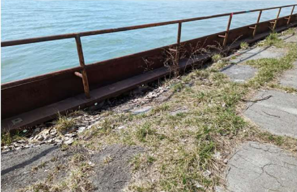
PHOTO 9: DETERIORATED ASPHALT, GRADE SLOPES TOWARD WALL
