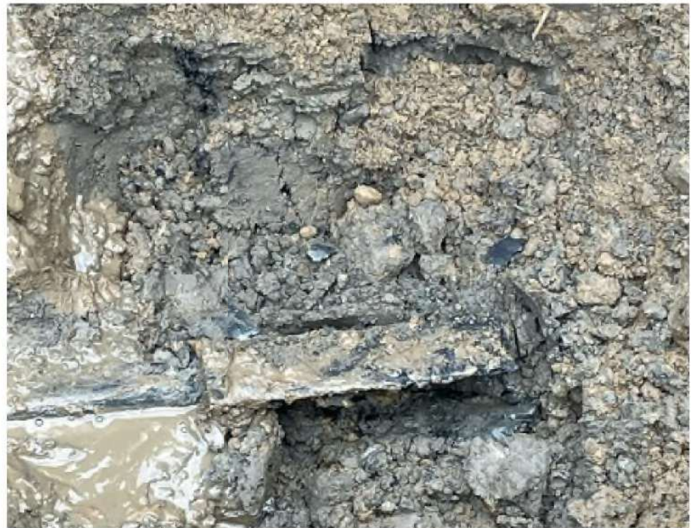
PHOTO 4: TERMINAL END OF EASTERNMOST TIEBACK- ANGLE MAY BE A TURNBUCKLE, BUT NO ROD WAS OBSERVED BEYOND 15' OFF BACK FACE OF SEAWALL, ROD ABOUT 5 FEET BELOW TOP OF SEAWALL.
