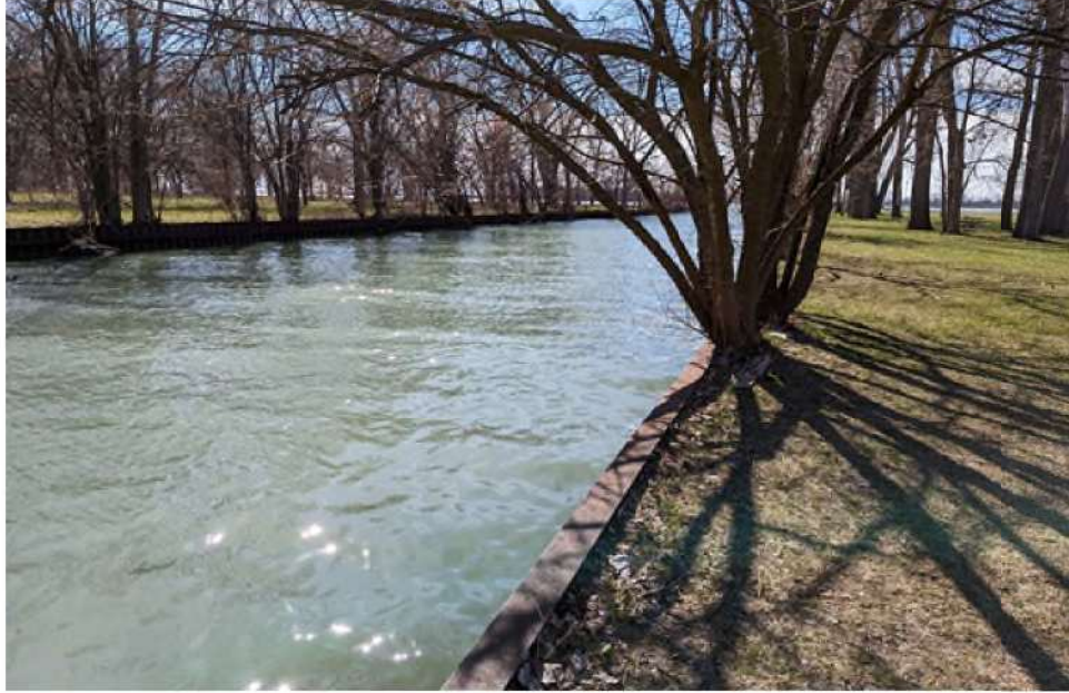
PHOTO 10: TREES BEHIND WALLS ARE DAMAGING WALLS
