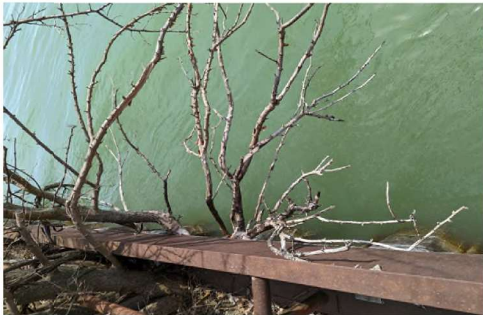
PHOTO 7: SCRUB AND ROOTS GROWING THROUGH WALLS, TIES EXPOSED
