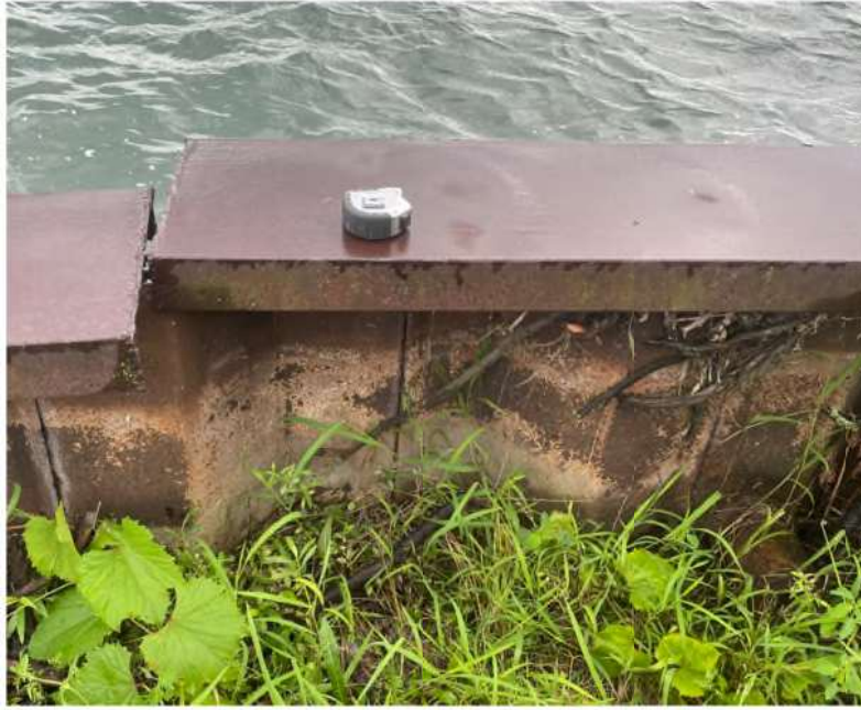
PHOTO 1: SEPARATION AT PILE CAP JOIN
