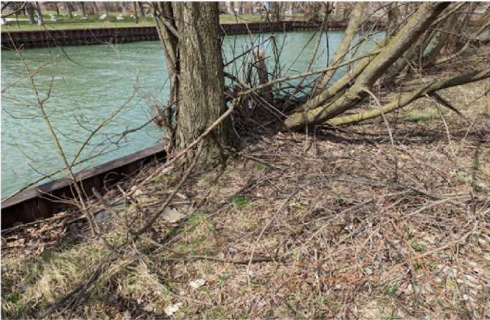
PHOTO 4: TREES HAVE RESULTED IN DAMAGE TO WALL
