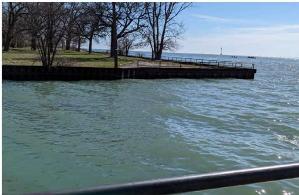
PHOTO 5: TREES BEHIND WALLS HAVE DAMAGED WALLS
