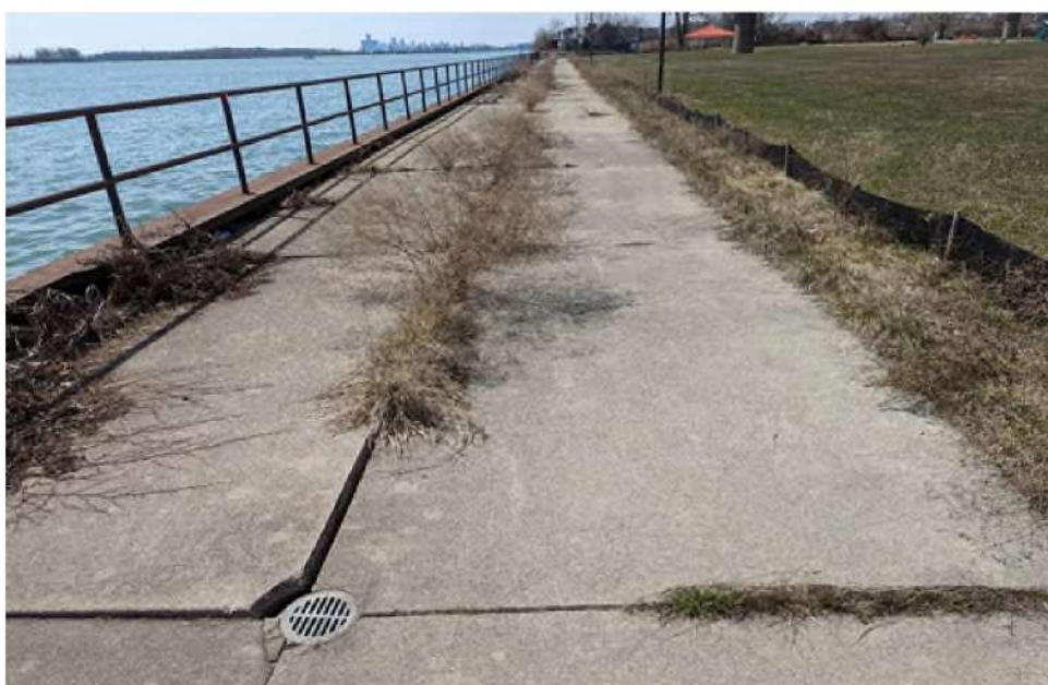
PHOTO 14: SIDEWALKS HAVE NOT BEEN MAINTAINED. NOTE SETTLEMENT, UNEVEN SLABS, SCRUB IN JOINTS
